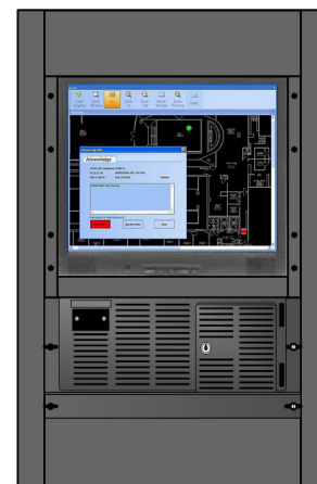
Figure 5: Rackmount PC and Monitor
